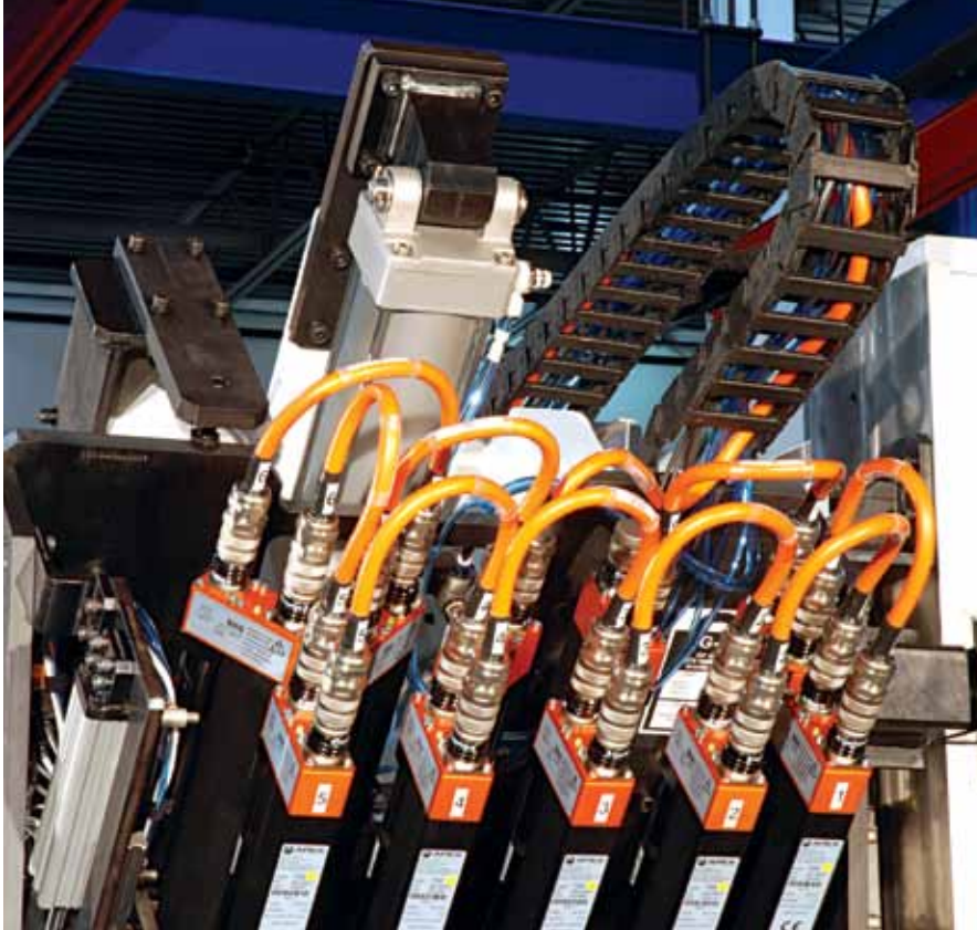
Shown above is a ten Intelligent spindle application with nine jumper cables and a single field cable that terminates at the power distribution box.
